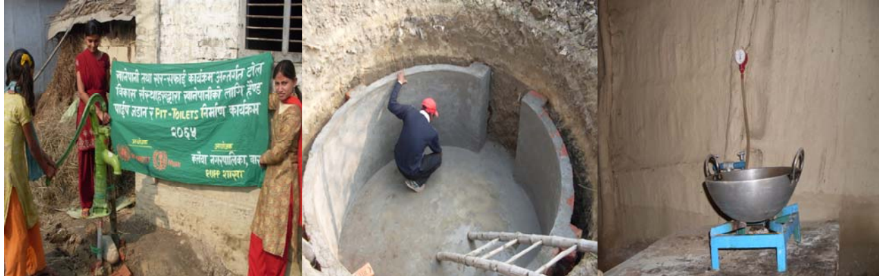
Progress on Kalaiya Project at various selected TLOs. 1) Hand-Pump Constructions and its inauguration by the locals (Left); 2) Pit-Toilet constructions with biogas (Middle); 3) Biogas implementation at Local kitchen room (Dishu)
